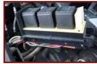
The EEC relay and the fuel pump relay (the two on the left) are car-killers if they fail. Ford did a good thing sequestering them in this neat little box.
